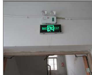
Photo of fire safety equipment Emergency exit.JPG
