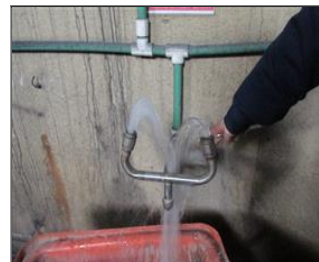
Photo first aid facilities Eye washer.JPG
