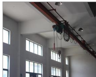
Photo of non-conformity NC-No safety latch was installed for the hook of the electric hoist.JPG
